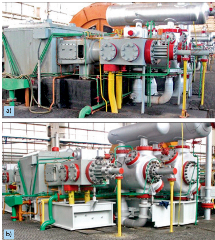
Fig. 6.50. Overall view of a 6HGP/4 reciprocating synthesis gas compressor: a) before modernization; b) after modernization of its seating arrangement
