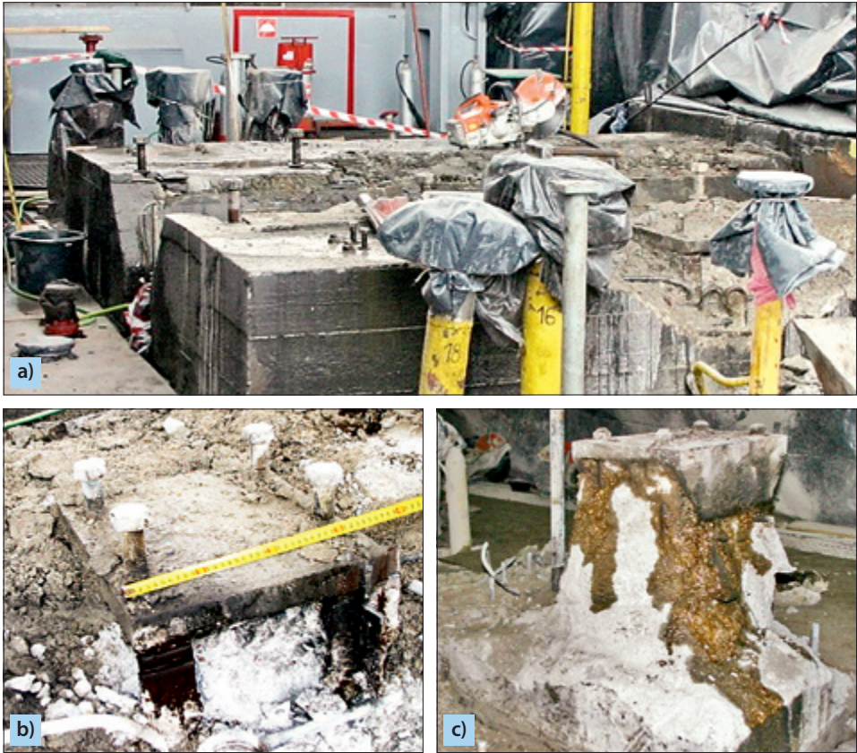
Fig. 6.43. An example of complete damage of the upper part of foundation of a reciprocating compressor with visible package of loosened sheets close to foundation bolts (a) and deep cracks in concrete and oil leakages (b, c)
