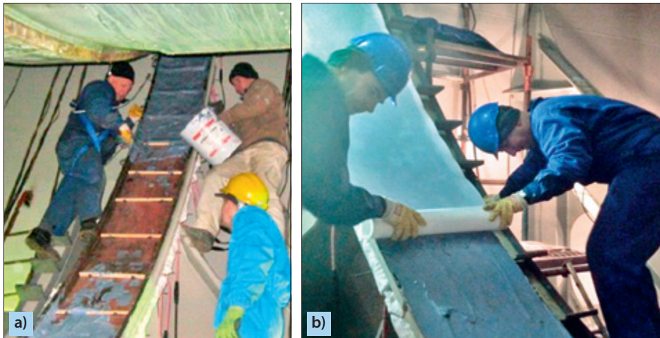
Fig. 6.31. Fragments of the performed assembling operations showing the spreading of compound over the tank support (a) and the covering of compound surface with Teflon film, after the spreading (b)
