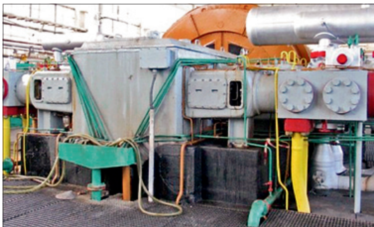
Fig. 6.41. Overall view of a reciprocating synthesis gas compressor (of 6HGP/4 type) traditionally seated on concrete foundation
