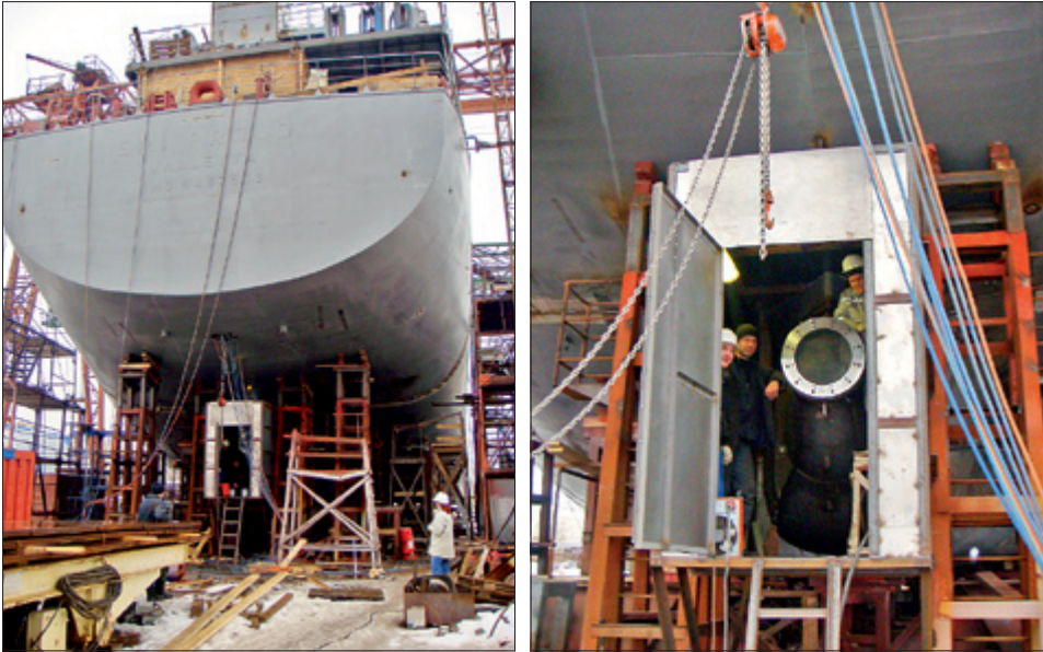
Fig. 5.19. Stern tube assembling in winter conditions with the help of a special booth heated with warm air (Onega Shipyard, Petrozavodsk, Karelia)
