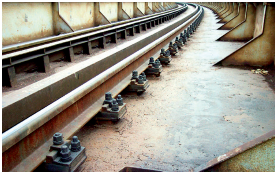
Fig. 6.70. An example of use of EPY compound for the seating of railway track on a steel over-bridge (in Szczecin)
