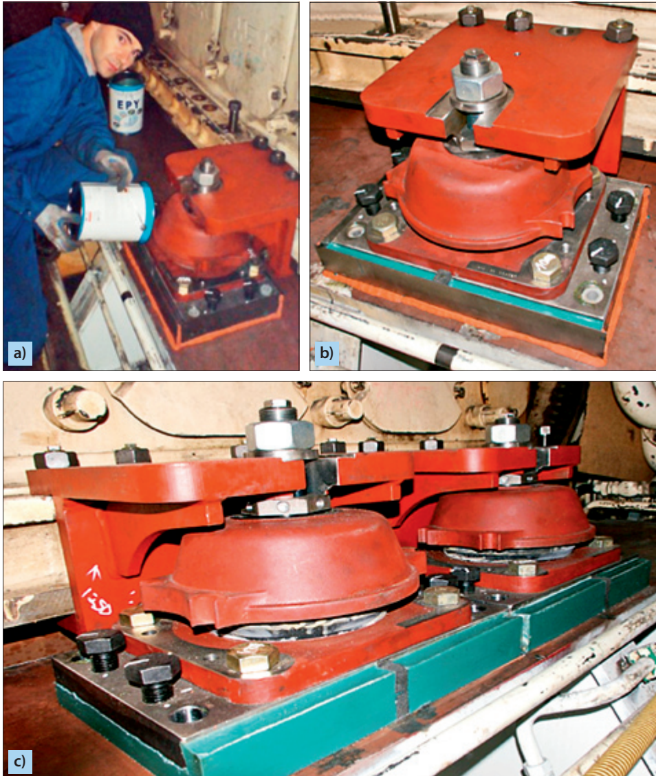
Fig. 6.7. EPY compound foundation chocks under shock absorbers supporting main engine of sea-going ship: a) filling the casting mould; b) the mould after filling with compound; c) ready-to-use chocks after removing the mould
