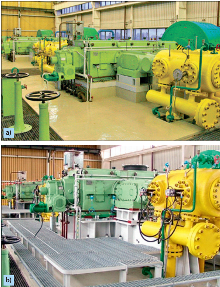
Fig. 6.49. Overall view of 1HB 5K-400/250 reciprocating compressors operating in natural gas pressing plants: a) before modernization; b) after modernization of their seating arrangements
