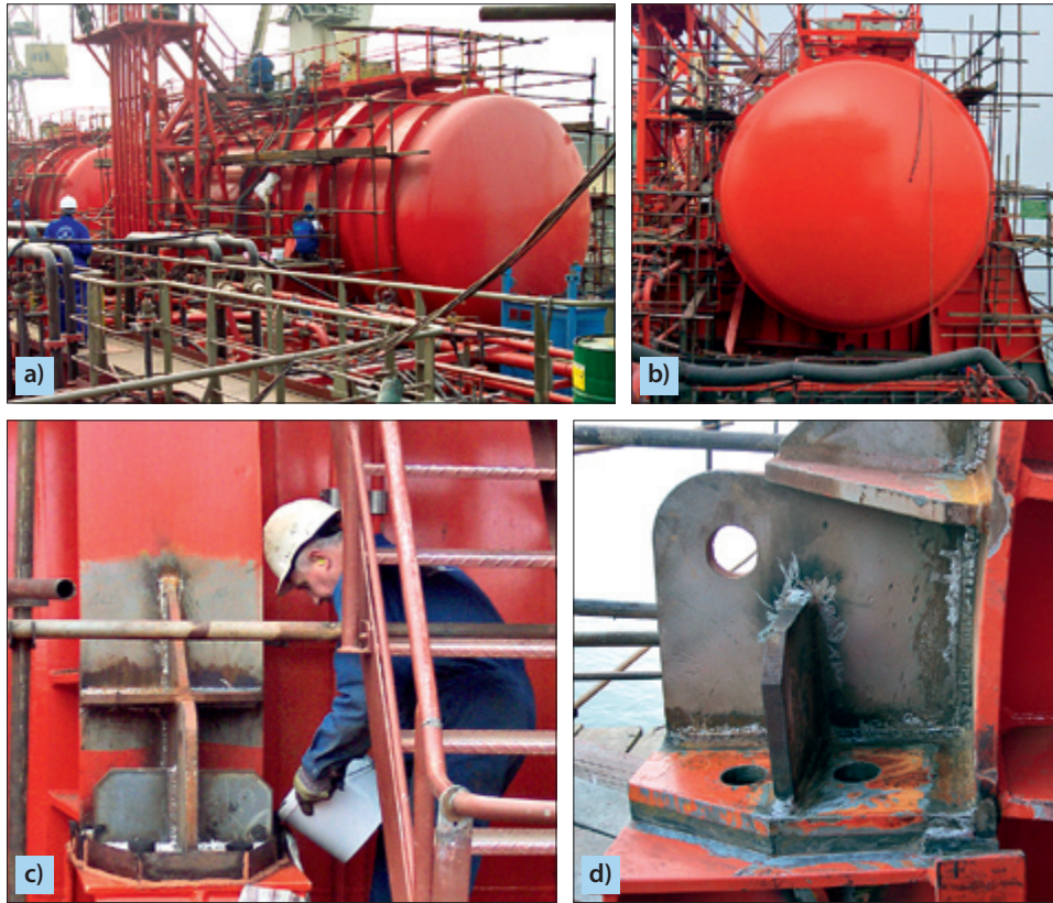
Fig. 6.25. Installation of the tank on the ship: a) and b) overall picture of the tank during installation; c) filling the pouring space with the compound; d) tank arm seated on EPY compound chock cast on upper flat surface of the bed
