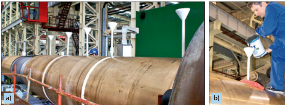
Fig. 6.17. The assembled unit prepared for filling with the compound (a) and a way of filling operation (b)
