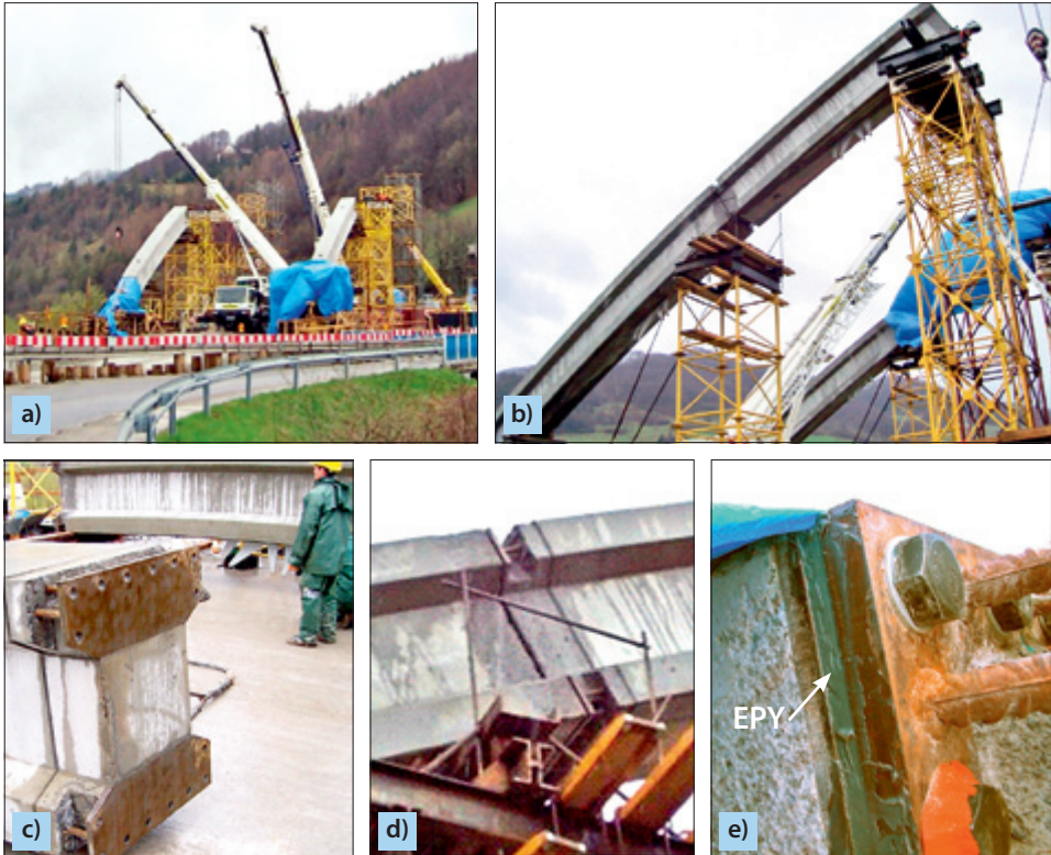
Fig. 6.71. Use of EPY compound in erecting reinforced concrete arc girders of a bridge built in Rytko, Poland: a) overall view of the bridge; b) a segment of arc girder; c) face connection surface of an arc girder segment; d) connection of two arc girder segments with visible gap to be filled with compound; e) a fragment of a multi-bolt joint with the gap filled with EPY compound
